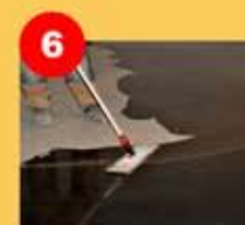
6 Application of the TERRACOAT and polishing for extra shine and sealing of the floor
